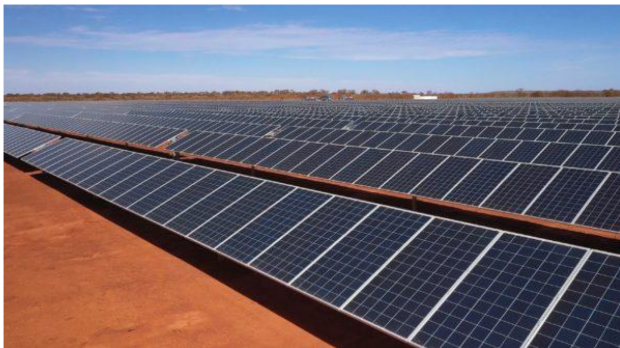
Figure 52 Granny Smith gold mine solar array 130
